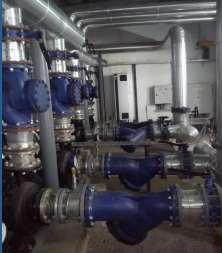
A view of Goktepe water pumping station
