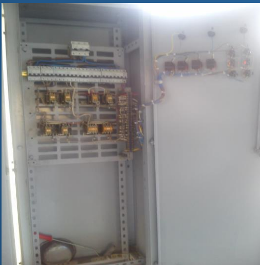
A view of Goktepe water pumping station
