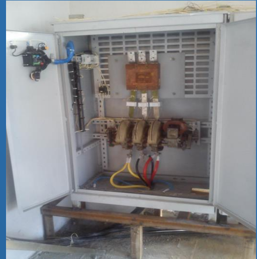
A view of Goktepe water pumping station
