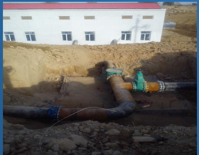
Sample Transfer Urban Water from Station Pumping & Construct Station Pumping
