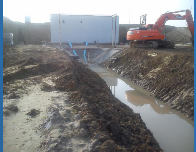
Sample Construct Station Sewage Transfer
