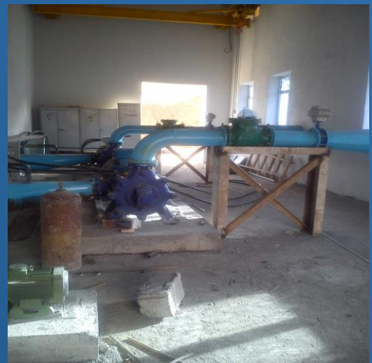
A view of Goktepe water pumping station
