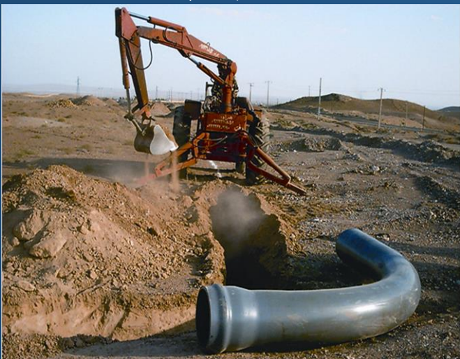
Pipe Water Transmission Line
